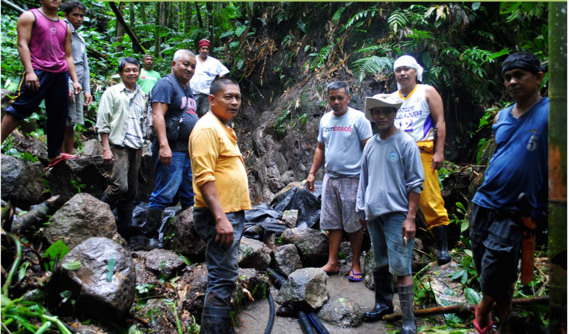
The spirit of volunteerism and "bayanihan" as villagers are installing a trial water supply system using a newly identified spring source.
